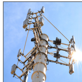
Cellular Base Station
