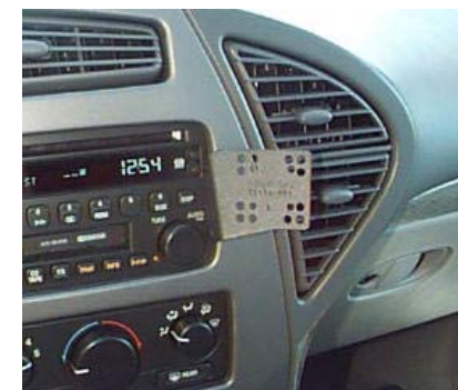
Finished install picture Rendezvous
