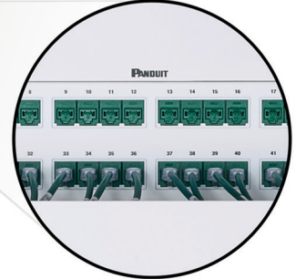
Block-Out Devices with Horizontal Cable Manager Patching
