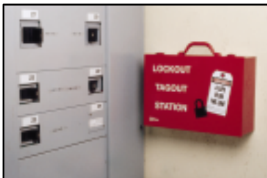
Mount close to power and distribution panels
