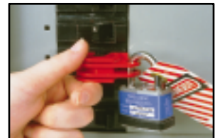
Verify that the lockout device secures the disconnect in a safe or off position.
