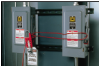
Lockout Single or Multiple Disconnects
